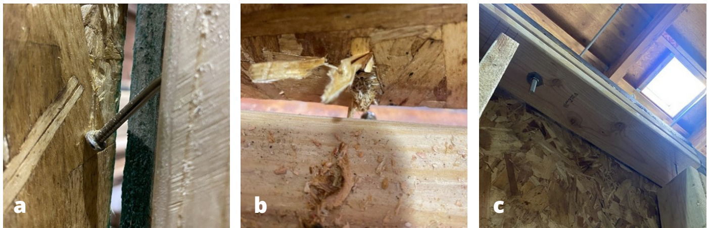
Figure 8. Observed failure types: (a) nail pull-out; (b) nail withdrawal; (c) stud-to-stud failure.
