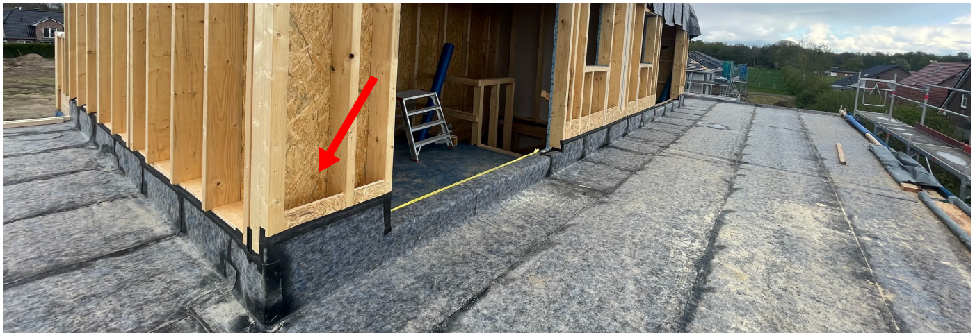
Figure 7. Incomplete protection with possible entrapment of moisture (author photograph).
