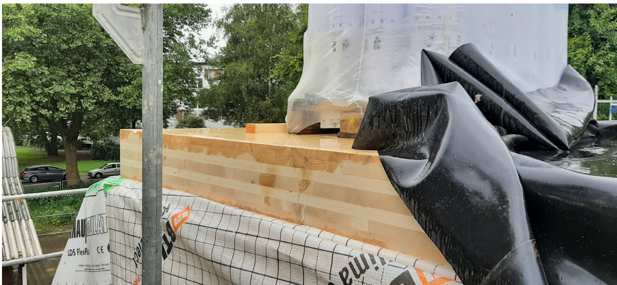
Figure 3. Storage of construction materials for the roof prevented the implementation of temporary weather protection measures (author photograph).
