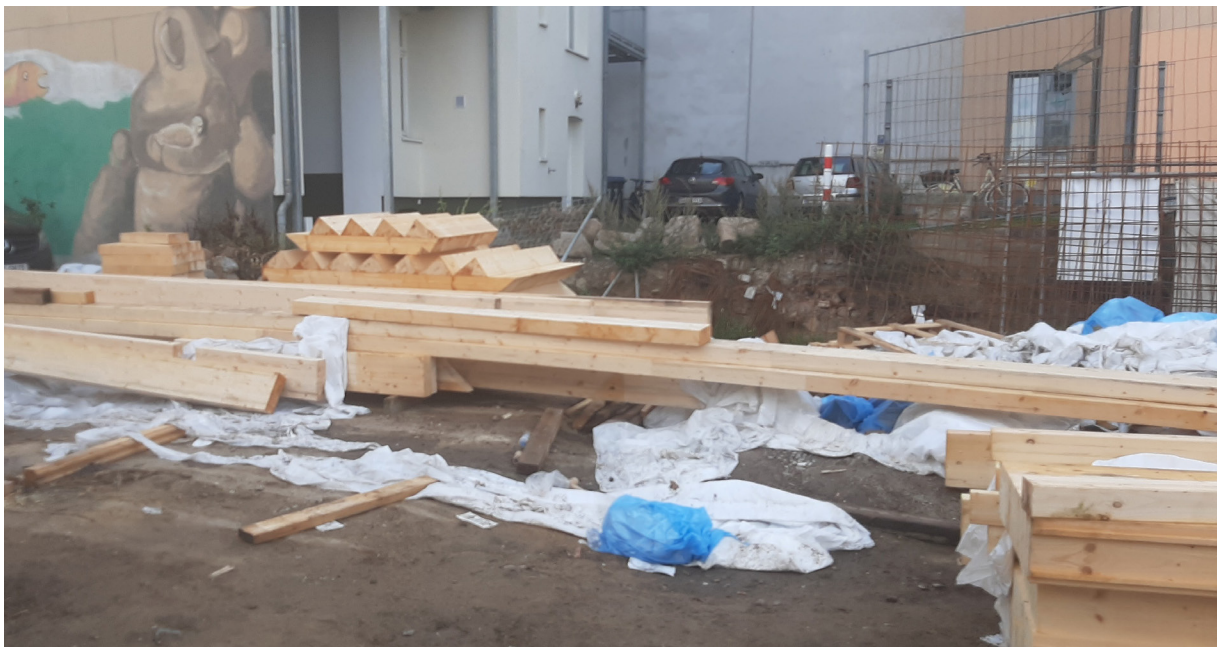
Figure 4. Disorganized construction site, inappropriate storing of mass timber elements (author photograph).
