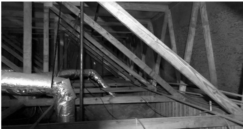
Figure 5. Series of repetitive flat roof trusses sitting on the exterior roof wall. Of particular interest is the unbraced 2 \times 4 compression web member running diagonally up from the exterior wall.
