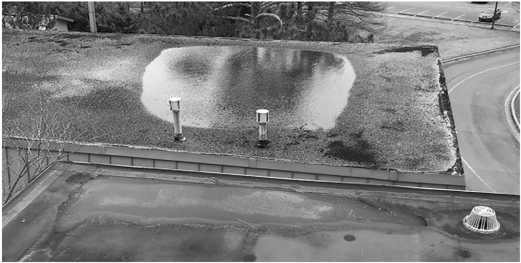
Figure 3. Ponding on roof, over an estimated 6.7 \times 6.7 m ( 22 \times 22 foot) area, hours before a heavy rain and windstorm event during which the roof collapsed.
