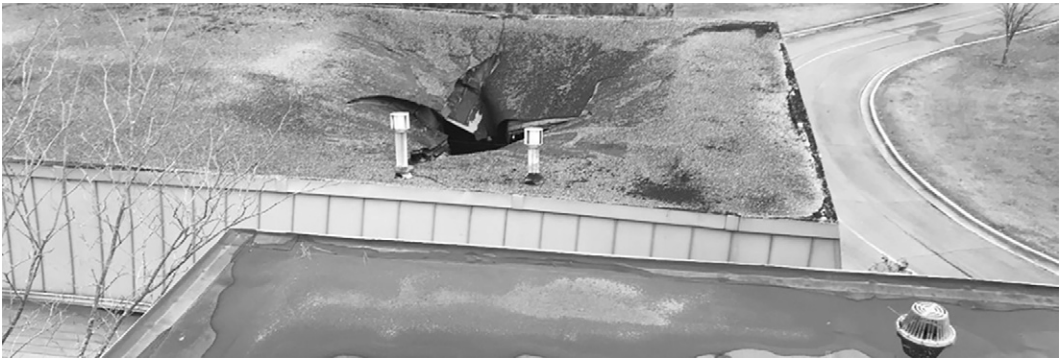
Figure 4. Roof section, approximately 7.3 \times 8.5 m ( 24 \times 28 feet), (7 trusses each 28-feet long) immediately following collapse.
