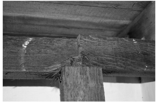
Figure 2. Crushing failure on a salt-damaged joist in the bilge of the Eureka .
